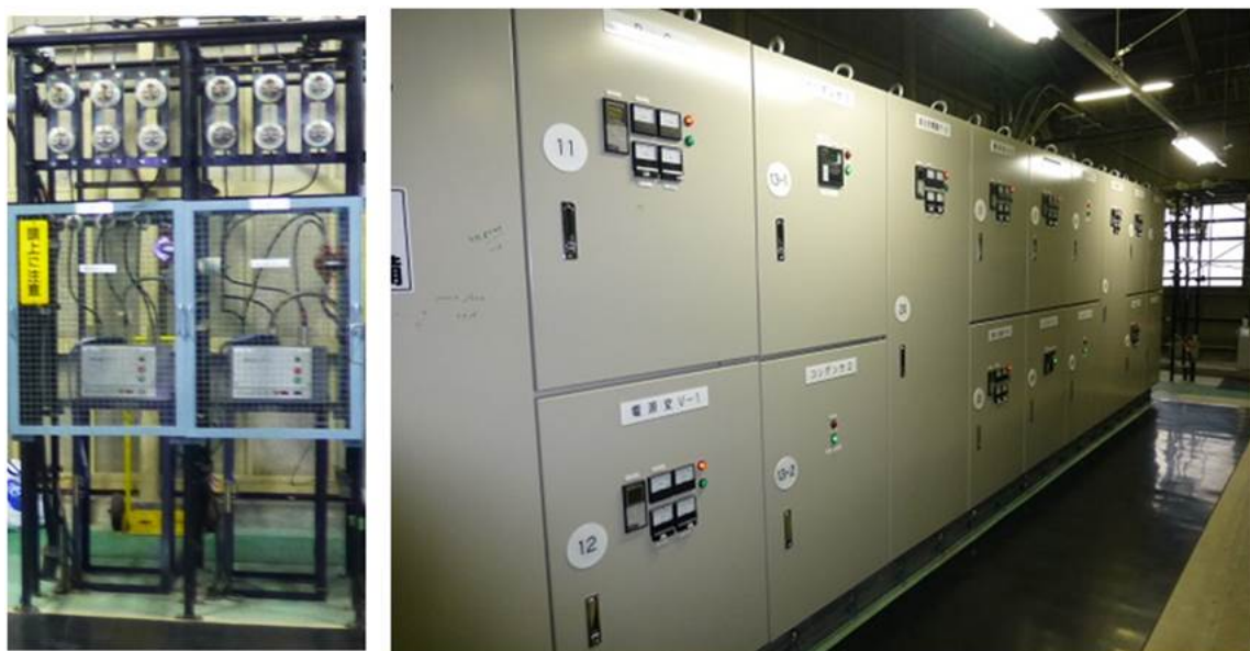
Fig.11. (left) Old switchboards, (right) new switchboards include vacuum circuit breakers (VCB) and protection relays. An automatic power factor controller is also installed in the new switchboard for proper control of the power system.
