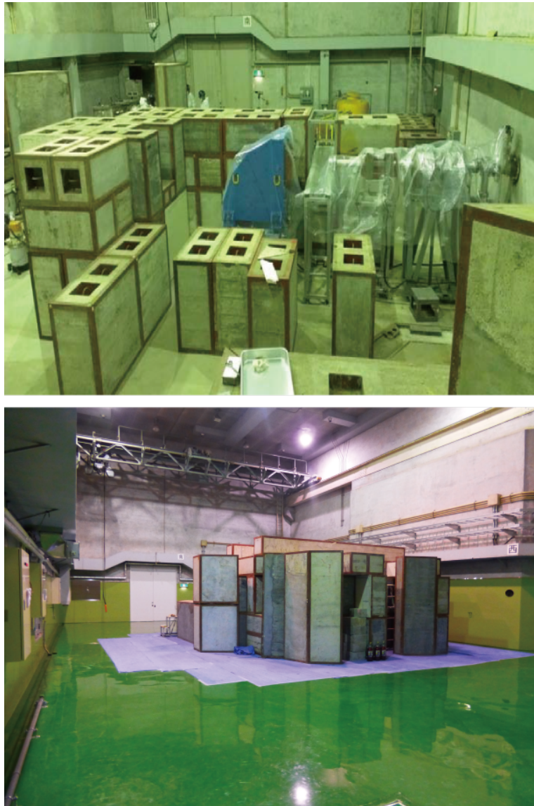
Fig.2. Renovation of wall and floor in the Exp. Hall No.1. Upper picture shows an end part of the beam line in the experimental hall before the renovation. Lower picture shows the reconstructed shield blocks after the renovation.
