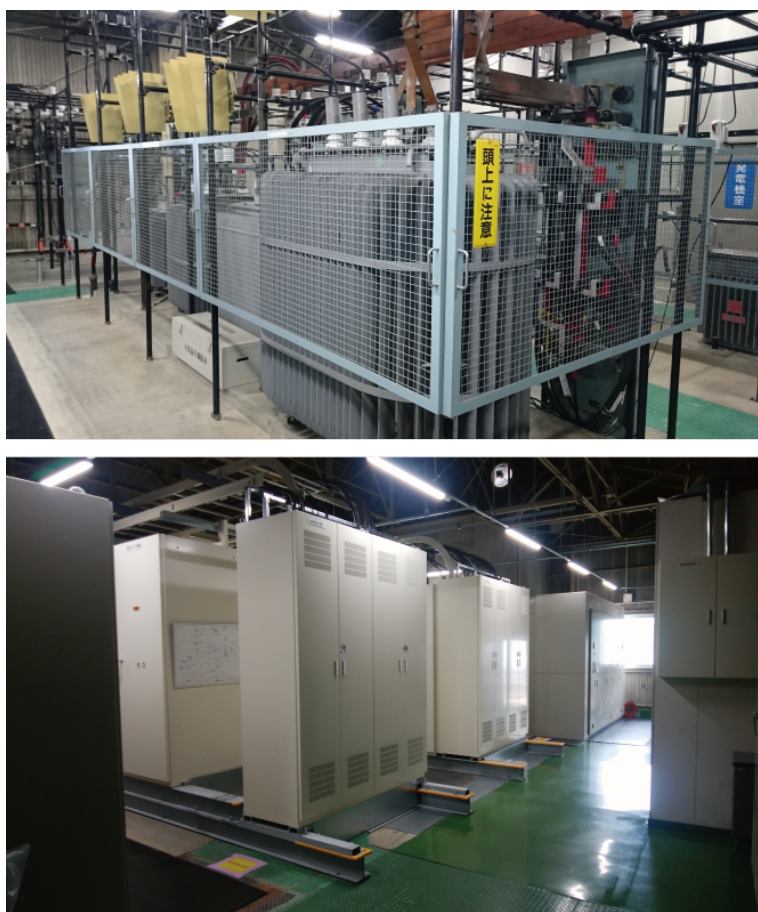
Fig.1. Transformers and switchboards in the indoor substation before (upper picture) and after the replacement (lower). The renovation of the indoor substation was also performed.
