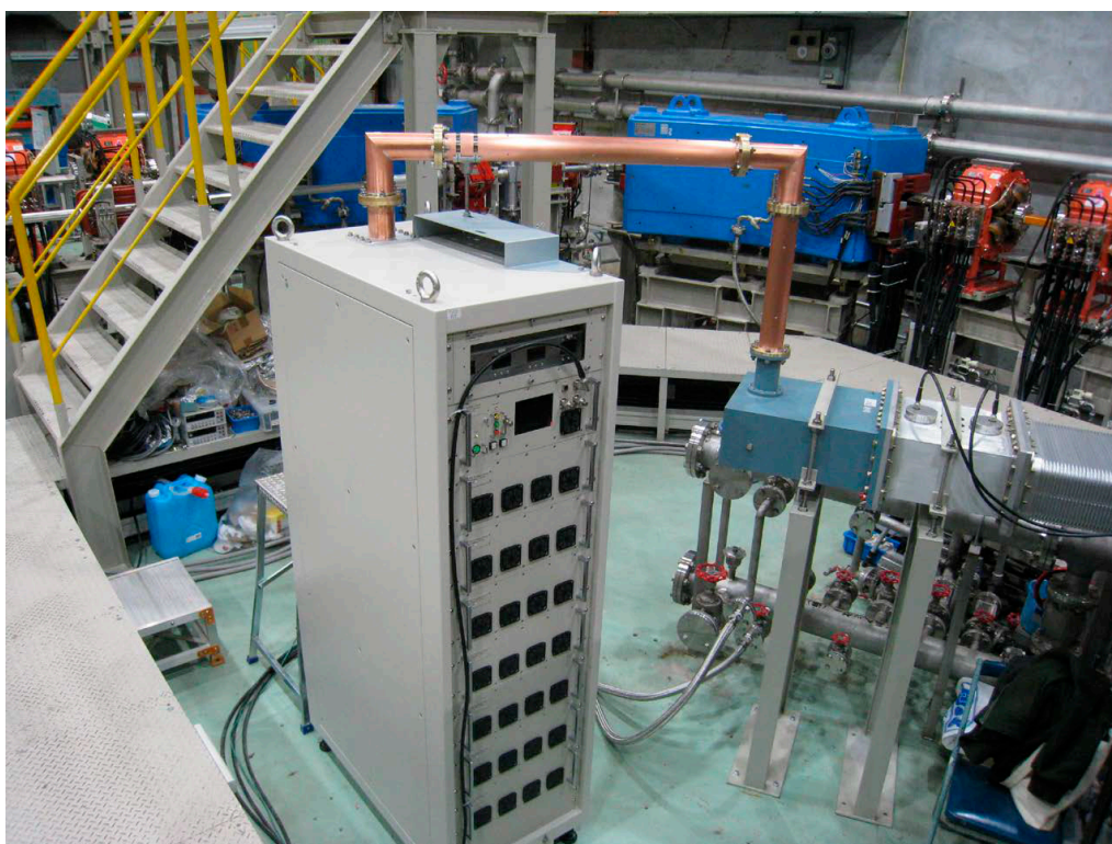
Fig.4. New RF power source installed to BST.
