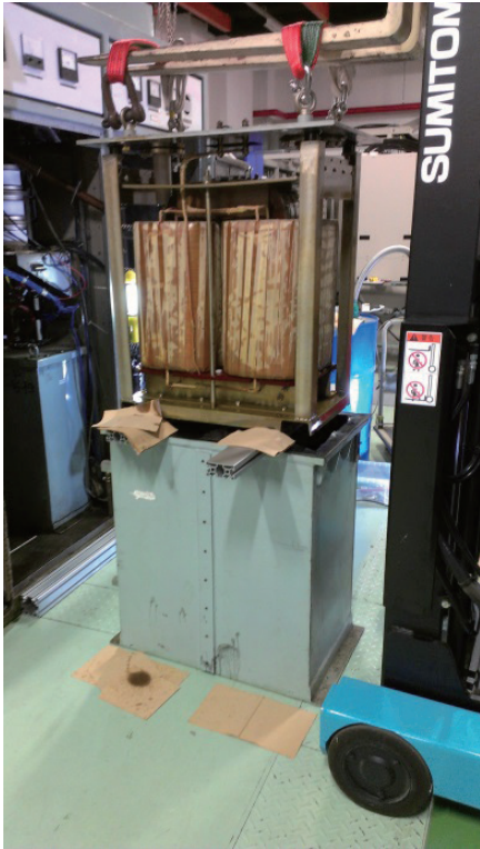
Fig.1. Voltage transformer extracted from insulation oil tank. It was cleaned and refilled with new oil.
