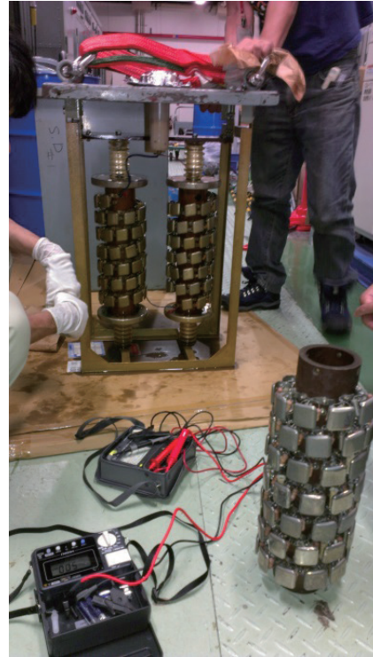
Fig.2. Voltage rectifier units extracted from insulation oil tank. The assembly which some elements fails (back), and re-assembled unit (front).
